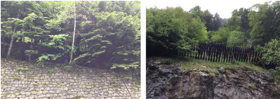
Figure 4.12. Retaining wall at the base of the slope, along the road (left), and protective fences, also near the base of the slope (right).
