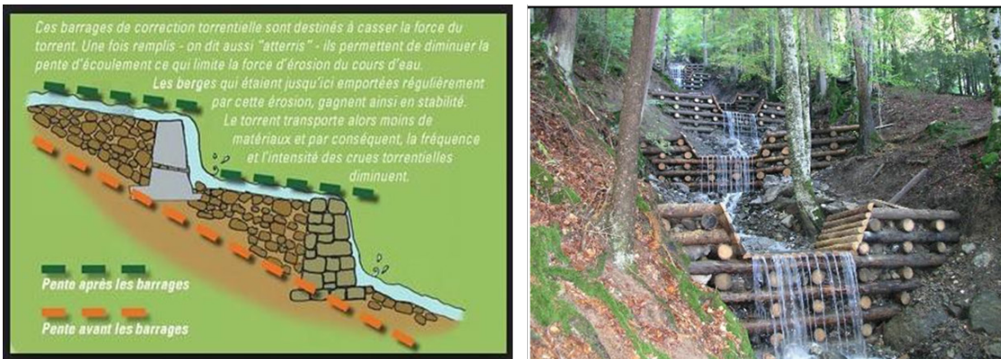
Figure 3.9 Principal sketch of the stepped solution with energy dissipating basins (left), and one possible solution sketched in the Socques proposal (right).
