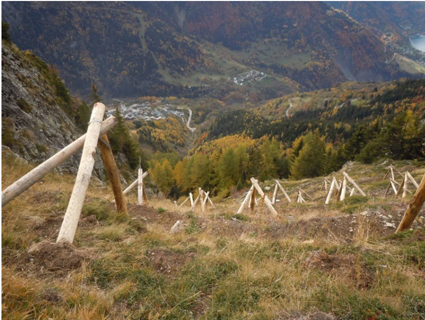
Figure 3.13 The type of wooden structures, made from local wood, planned for implementation to protect the plants from damage by snow creep during the first years. The structures will themselves also prevent release of snow avalanches.
