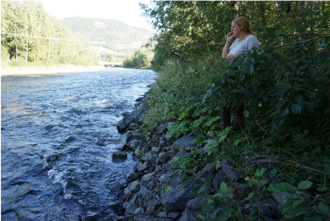
Figure 2.4 The base of the original (from 1995) 400m long barrier along the river Gausa. This barrier will be removed and replaced with one 100-250m inland.
