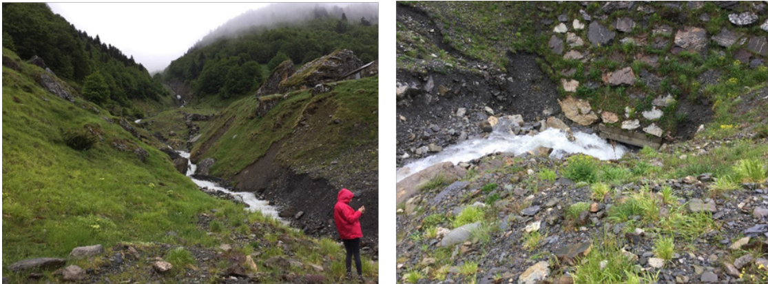
Figure 3.8 The ravine at Socques, seen from the road, upstream (left), with easily erodible sediments seen all along the ravine, and the nearly clogged culvert under road RdD-934 (right). The culvert dimensions are 3x4m.
