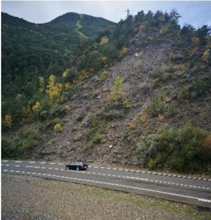
Figure 3.6 The problematic slope at Santa Elena.
