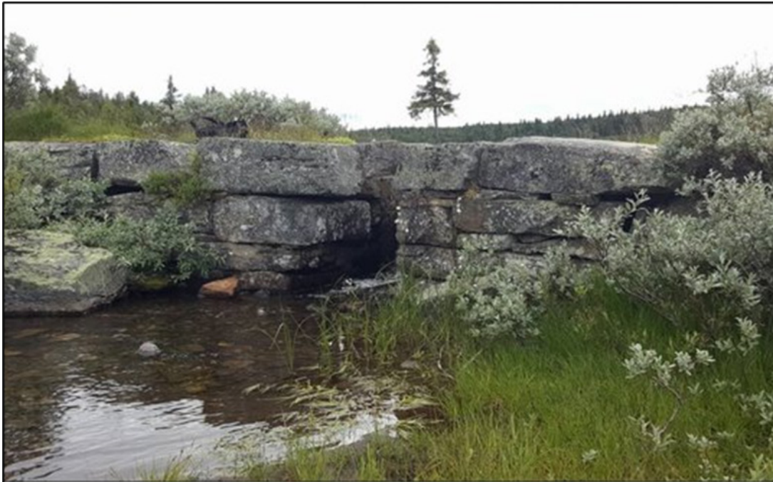
Figure 6-8 The existing old dam at Lake Svintjønna. The measures will increase the dam height by ca. 0.5 m and establish a new gate and threshold, with automatic monitoring of the lake level.
