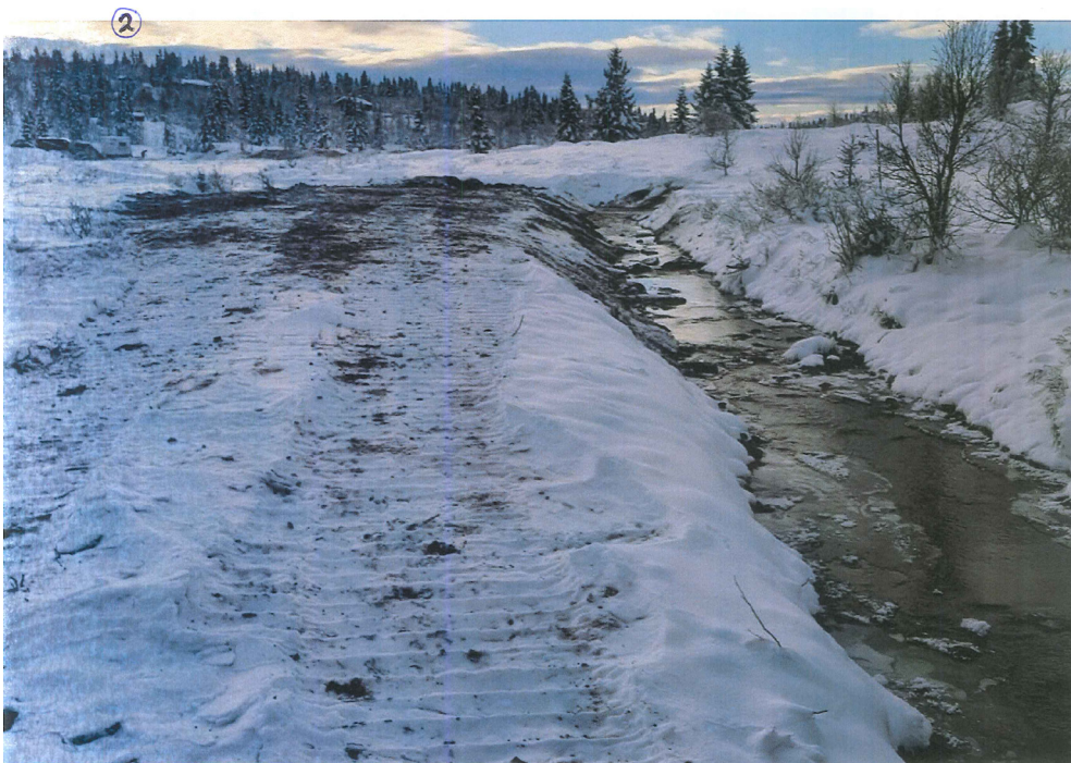
Figure 6-10 The new, deeper spillway from the Lake Svintjønna dam. (Photo: Ole Johan Kolseth)
