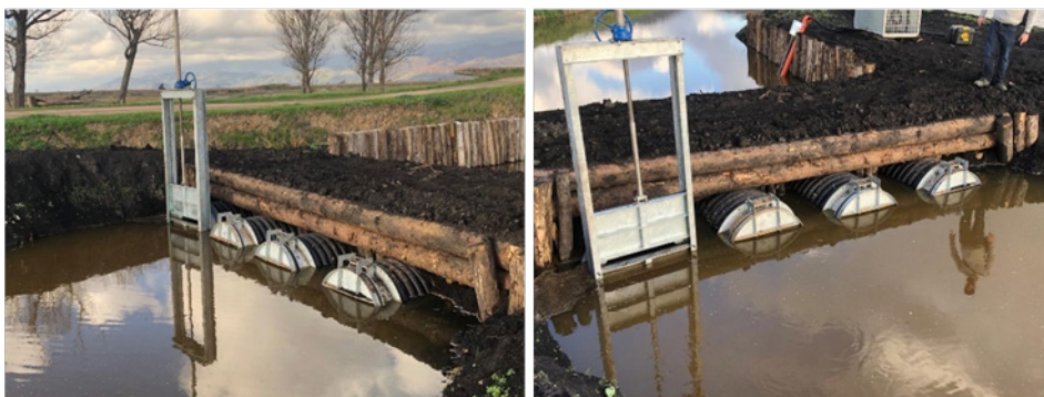
Figure 4-6 Photos of the pipes with clapet valves through the threshold (Figure 4-5) (Photo: ADBS)
