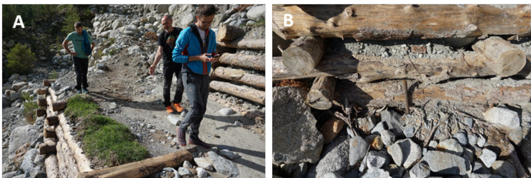
Figure 5-19A) Close-up of one of the terraces, with grass taken directly from one of the local pastures. All terraces will be planted with grass and other local bushes and trees. B) Close-up of the construction, anchored by iron rods, pushed at least 2 m into the ground.
