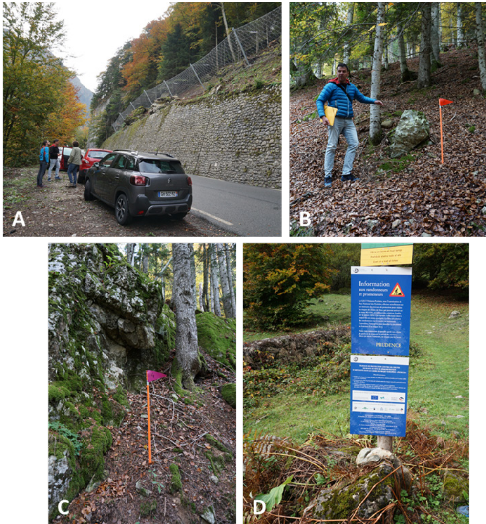
Figure 5-9 A) Newly established rockfall nets in one section of the slope at Artouste. B) A loose boulder, which is flagged to indicate type of protective structure to be implemented. C) Rock ledge, potential source of rock fall, flagged for NBS protective measures. D) Poster at the Artouste slope, informing about the project and the NBS measures to be implemented.
