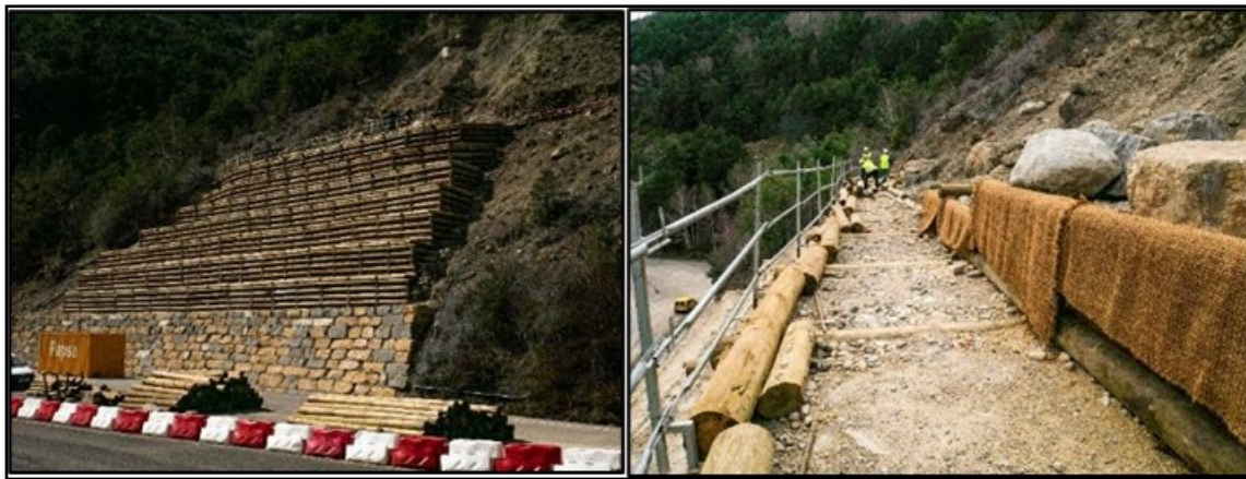
Figure 2. Work area in the Santa Elena roadcut. The monitoring area includes ten 2m wide gardeners of decreasing length (from 30 m for the lowest level to about 10m for the top level).
