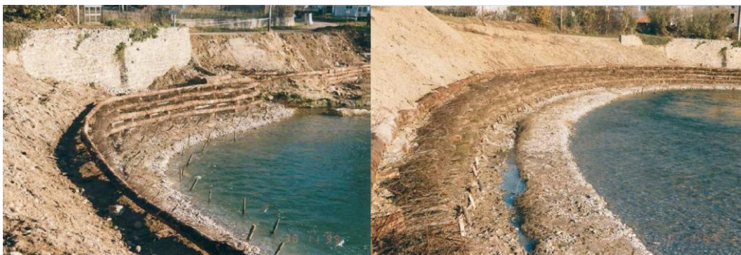
Figure 2-20. Example of fluvial slope stabilization in an urban area (Klaus Peklo, EFIB).
