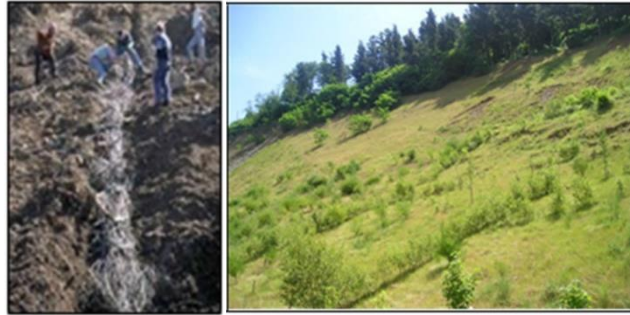
Figure 2-10. Stabilization technique. Construction on slope and in herringbone, in Bergara, Gipuzkoa (EFIB, Paola Sangalli).
