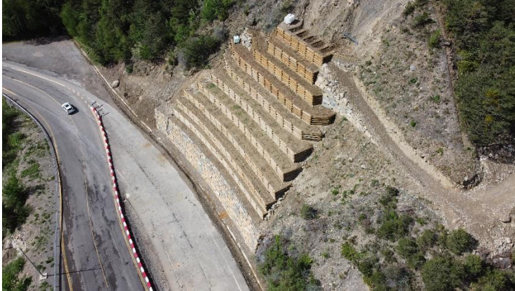
Figure 1-7. Overview on the site of Santa Elena, taken with drone, with the masonry wall and the wooden terraces at the end of the works.
