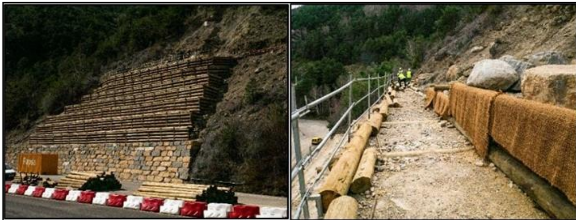
Figure 3-9. Work area in the Santa Elena roadcut. The monitoring area includes ten 2-m-wide terraces of decreasing length (from 30 m for the lowest level to about 10m for the top level).
